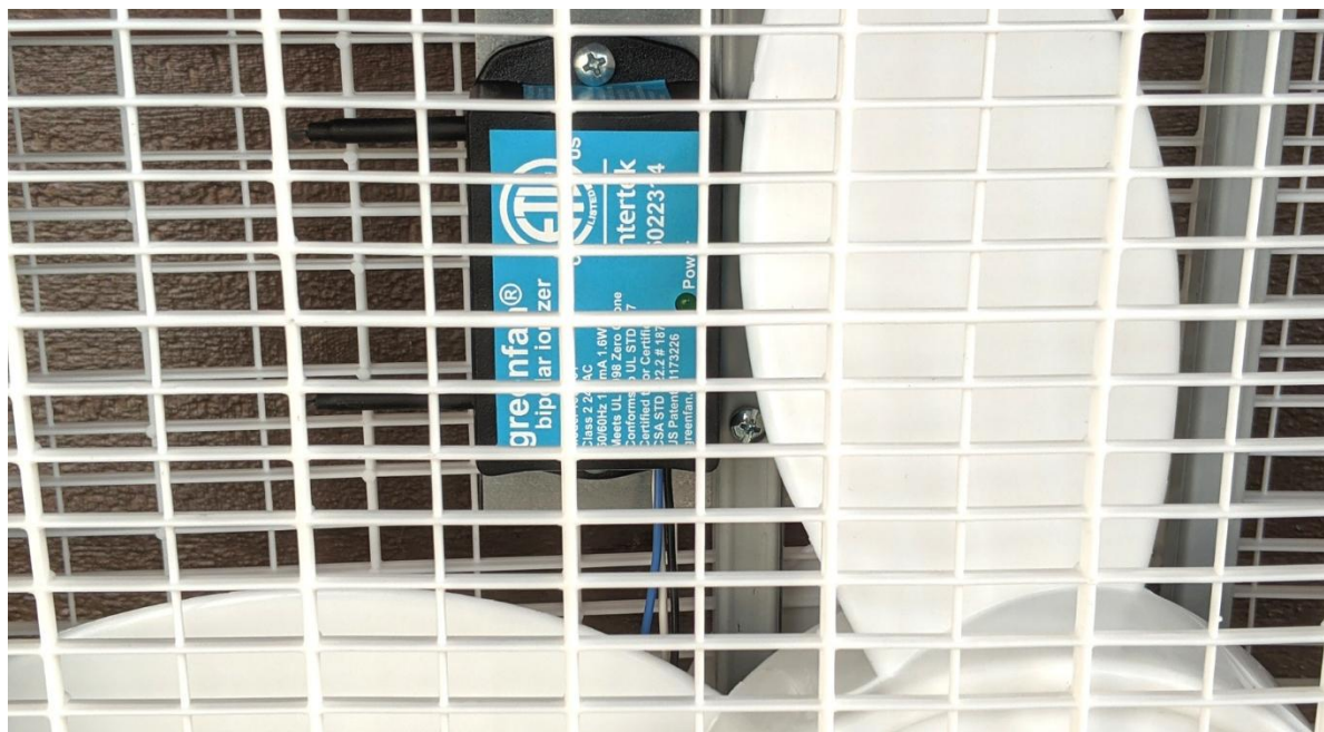
Figure 12. Bipolar ionizer installed at inlet of ventilation fan behind protective grill
